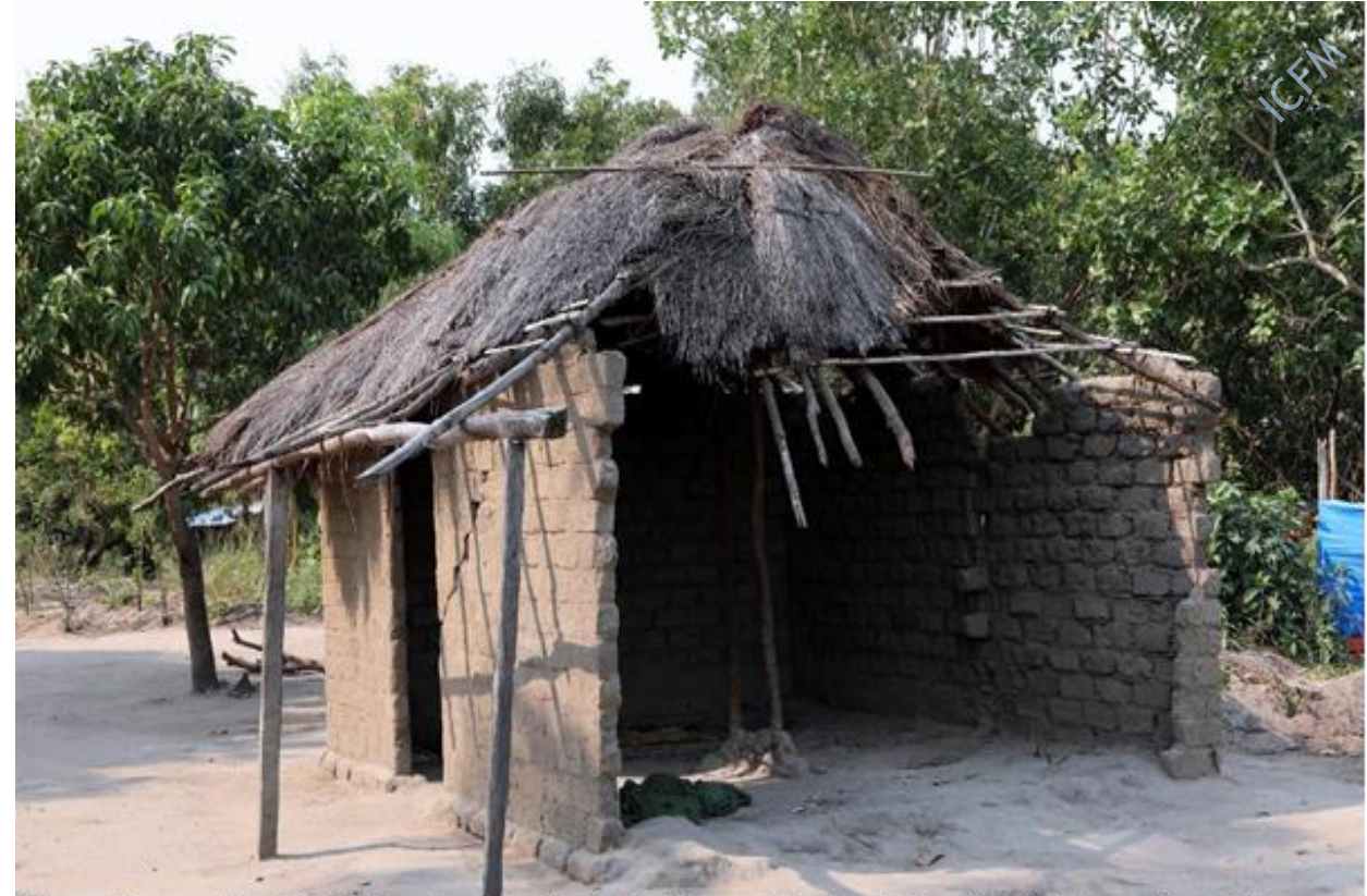
House damaged by Tropical cyclone Freddy in Quelimane, Zambezia Province in Mozambique. The proposed Recovery and Resilient building project will promote and support construction of more Cyclone resilient buildings for the poorest households in the affected countries
